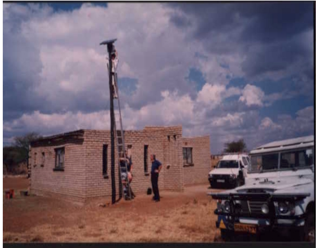
Telkom DECT domestic installation 30 watt module. Mafeking, South Africa.
