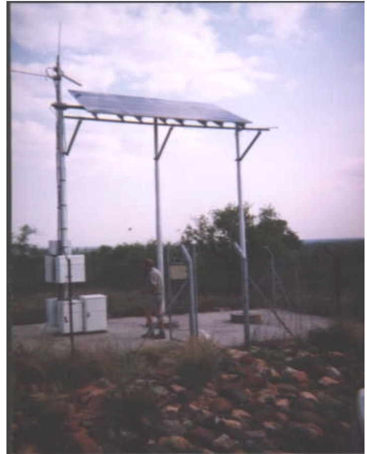
RurTel repeater station on game farm - Northern Province, South Africa.
