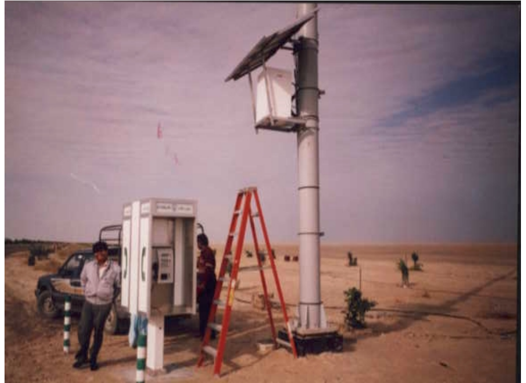
Etisalat emergency phone installation outside Abu Dhabi - in the desert.
