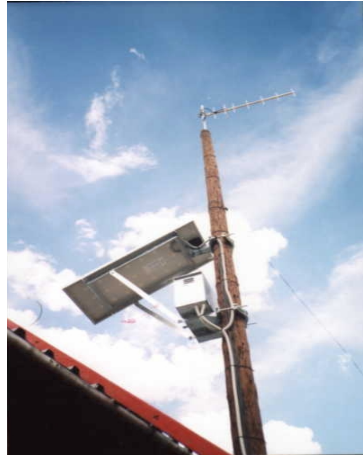
75 watt module powering a Siemens Ultraphone. Farmhouse in Namibia.
