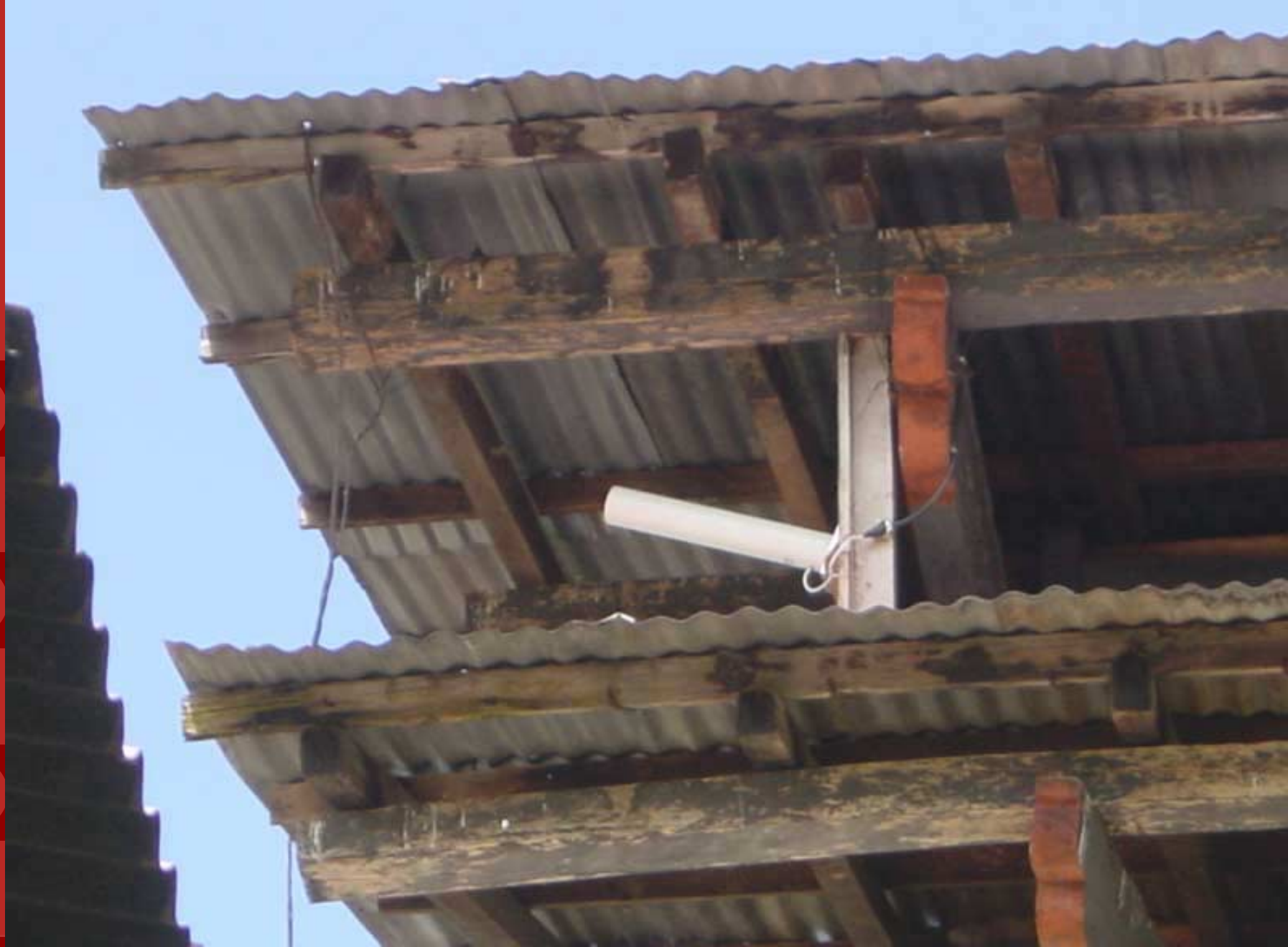
Closeup of Yagi Antenna
