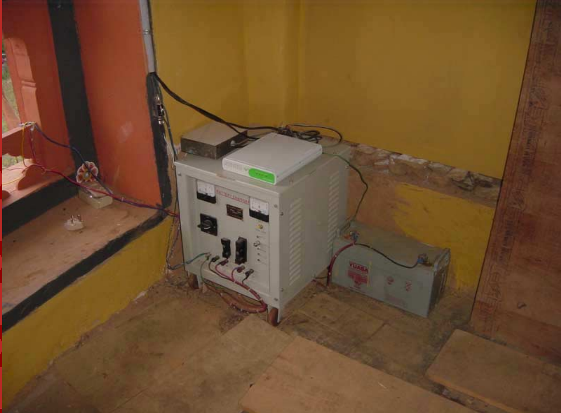
Power supply, VOIP gateway, 802.11b client 38
