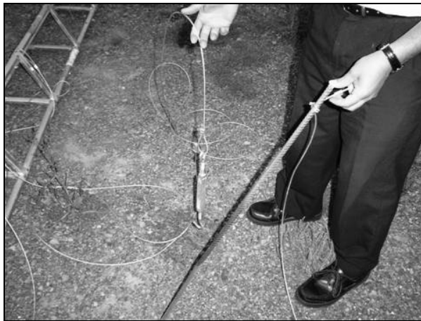
Photo 13-1: Guy Wires and Turnbuckle
