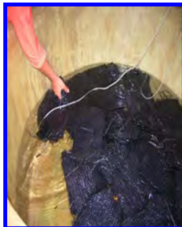
Kolektor didalam fiberglass
