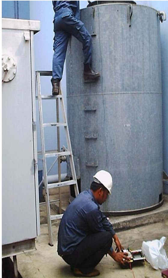
Gambar 3.21. Pengukuran Neutral Grounding Resistance
